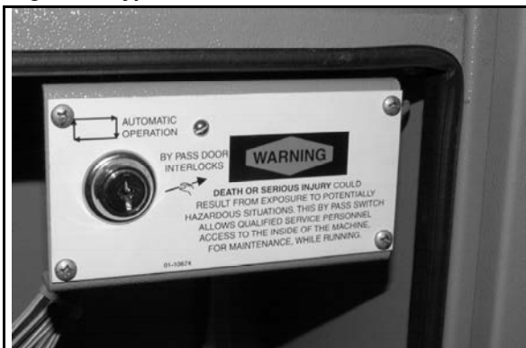
Figure 1: Bypass door switch
