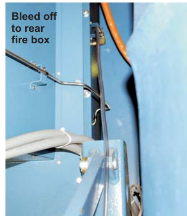
Bleed off to rear fire box
