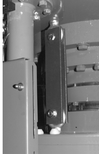
Figure 1. Safety Bars Deployed
