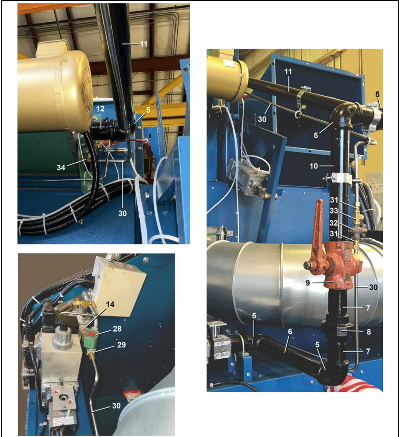
Figure 35. Gas Train and Pilot Line
