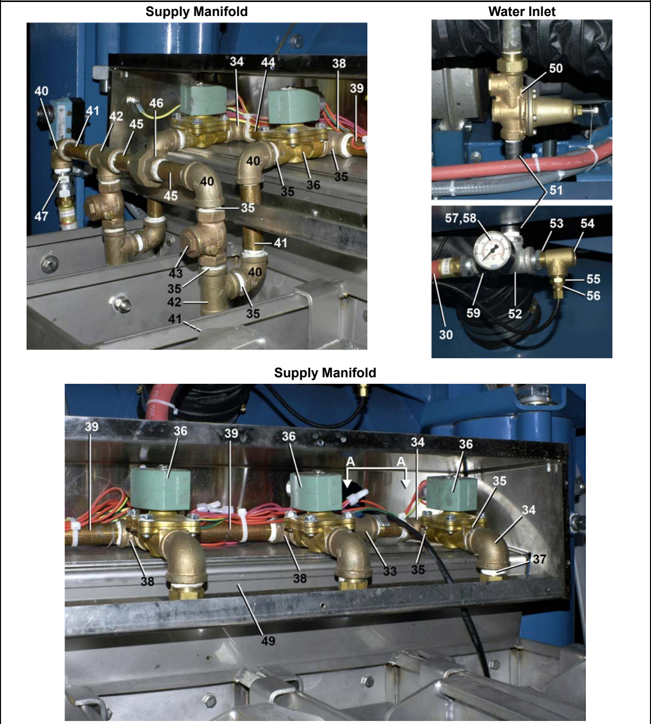
Figure 69. Water inlet and manifold piping
