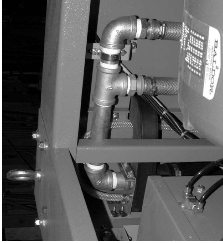
Inlet for Peristaltic Chemical Supplies See BMP040050.
