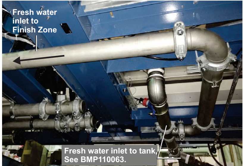
Bottom View Manifolds
