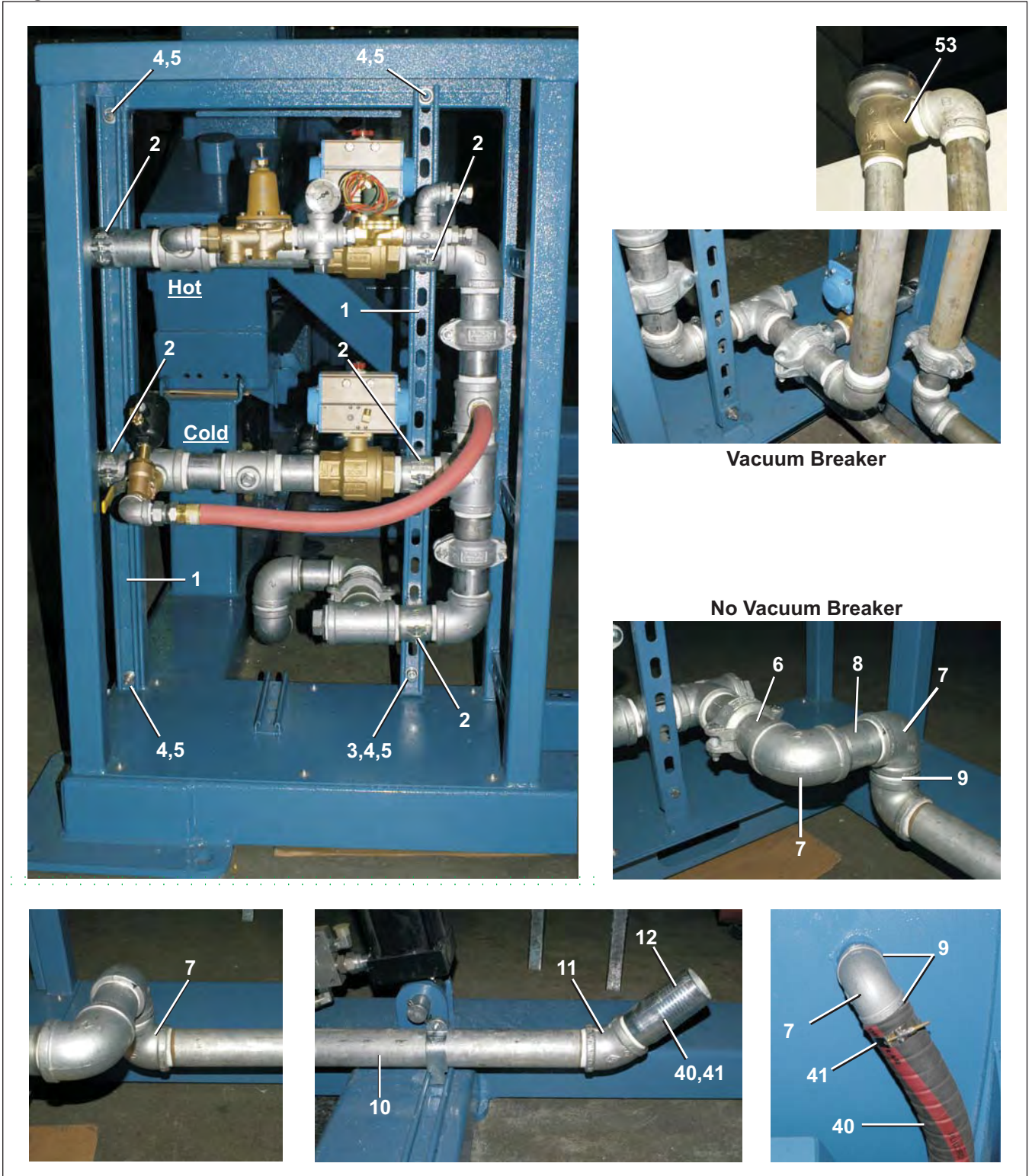
Figure 1: Water valves installed
