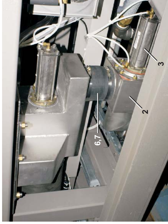
(C) Drain Stop: Flow Not to Sewer
