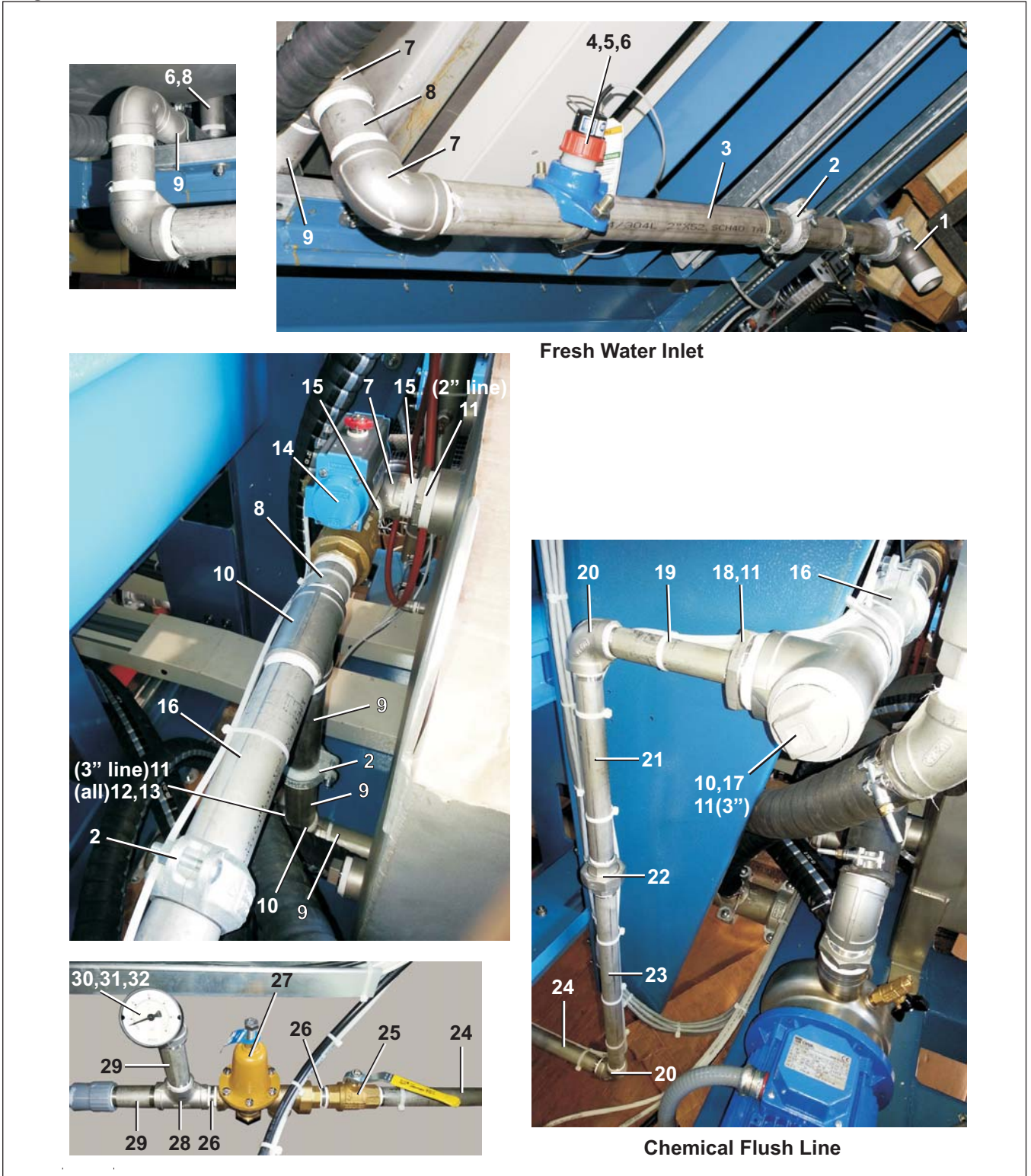
Figure 1: Fresh Water to Tank
