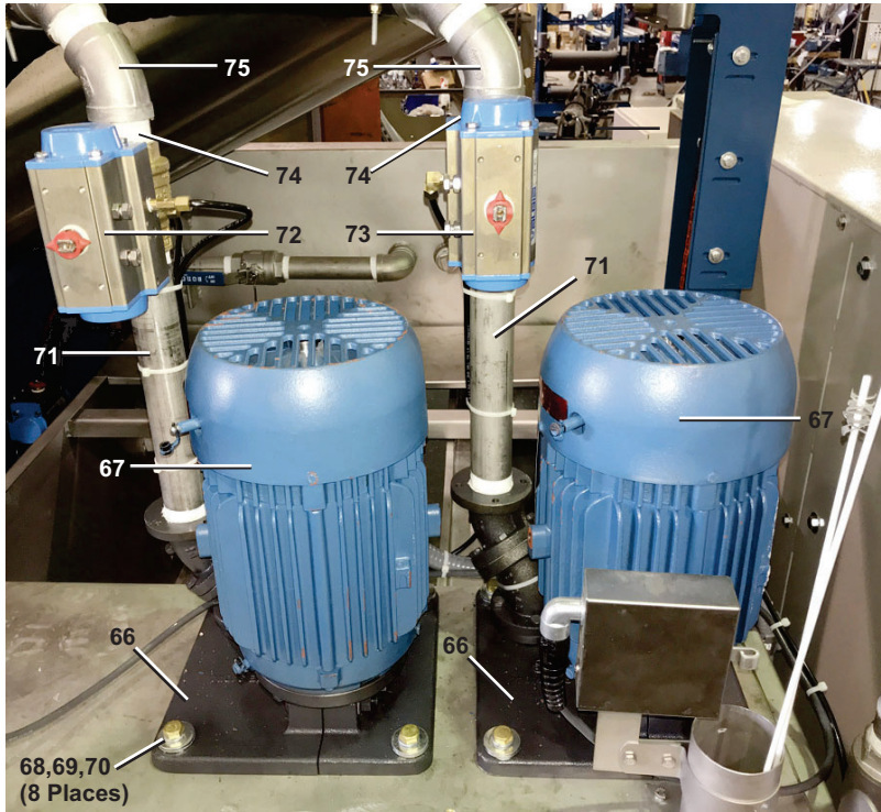
Figure 4: Pumps, Valves, Probes, and Sensors
