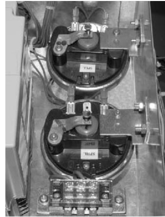
Two Level Switches Used
