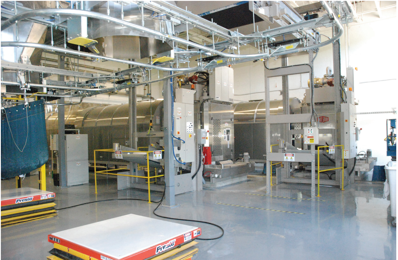
FULL COMPLEMENT: The plant featured two 150 lb (68 kg) 10-module PulseFlow technology tunnels, 10 Milnor 64064 gas dryers arranged in a pod configuration, three 170 lb (77 kg) Milnor dryers, and three 170 lb (77 kg) Milnor washer-extractors, as well as an automated rail system and flatwork finishing
