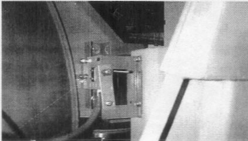
Bracket for excursion switch is modified by adding one hole two inches below bottom hole.
