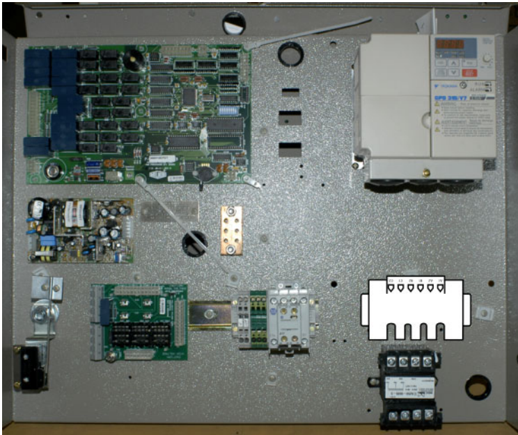
Figure 1: Typical Location for Inverter Reactor
